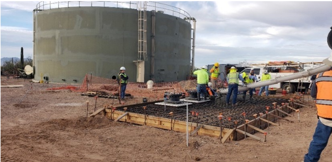
Smyth Industries is the general contractor constructing the Shannon Rd. reservoir and booster station. Construction is ahead of schedule and on budget.
