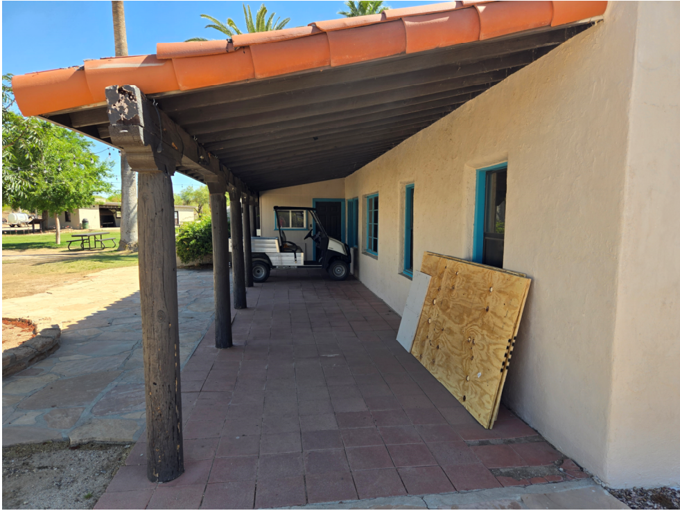
Photo 7: Wood rot at entry porch
