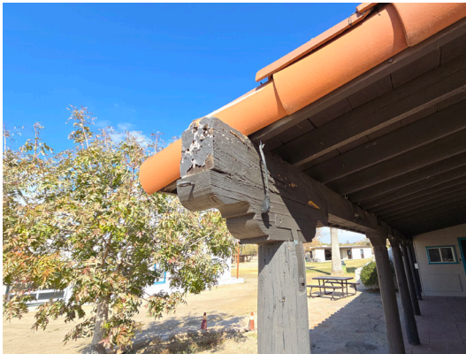
Porch beam with visible wood rot
