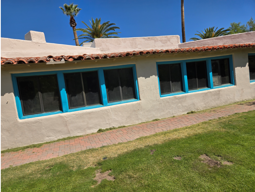
Photo 3: Deflected headers at Arizona room (note deflection in roof)
