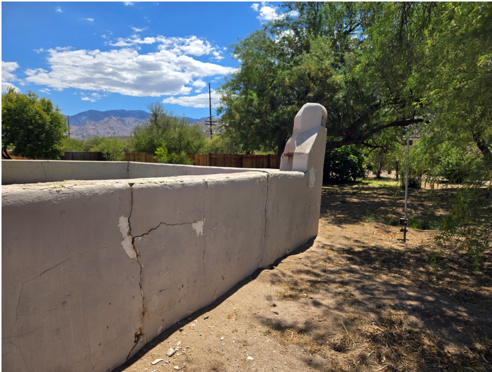
Photo 8: Deterioration of existing site wall and barbecue
