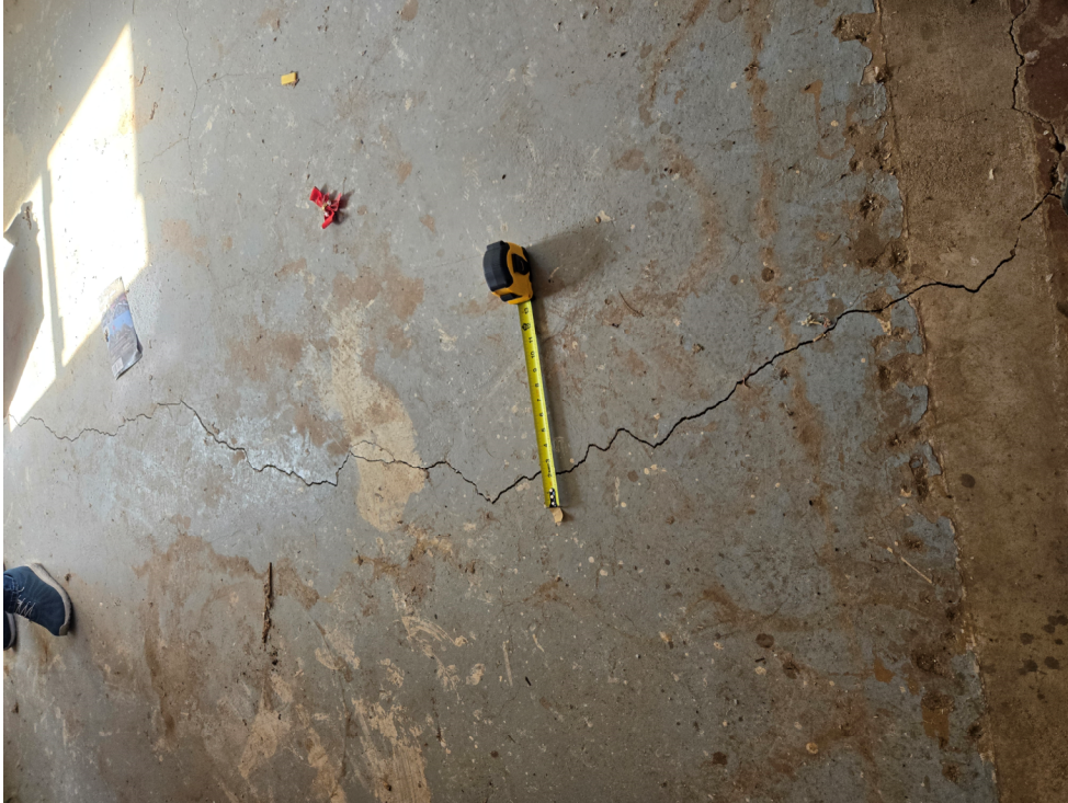
Photo 1: Typical cracking at slab on grade (note lack of joints)
