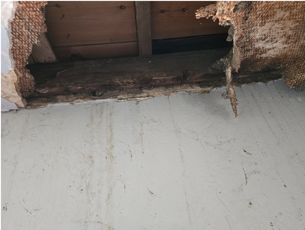
Photo 6: Water intrusion and water damaged wood framing
