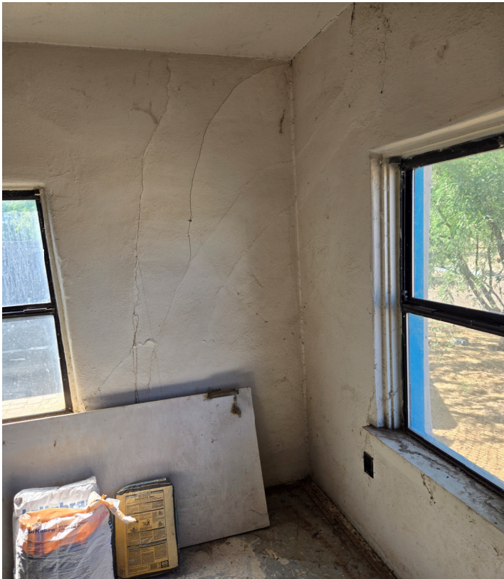
Photo 4: Typical cracked plaster at interior of existing adobe wall
