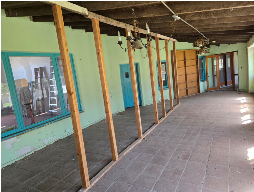
Photo 2: Shored deflected roof joists at Arizona room
