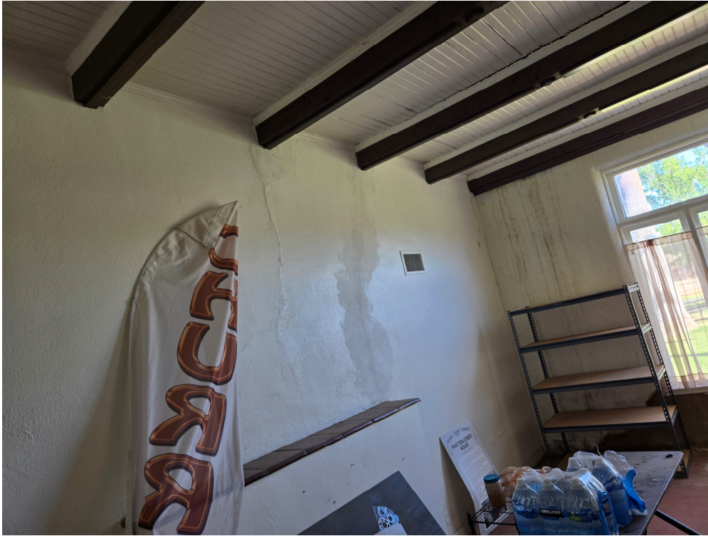
Photo 5: Water intrusion and plaster cracks at adobe walls
