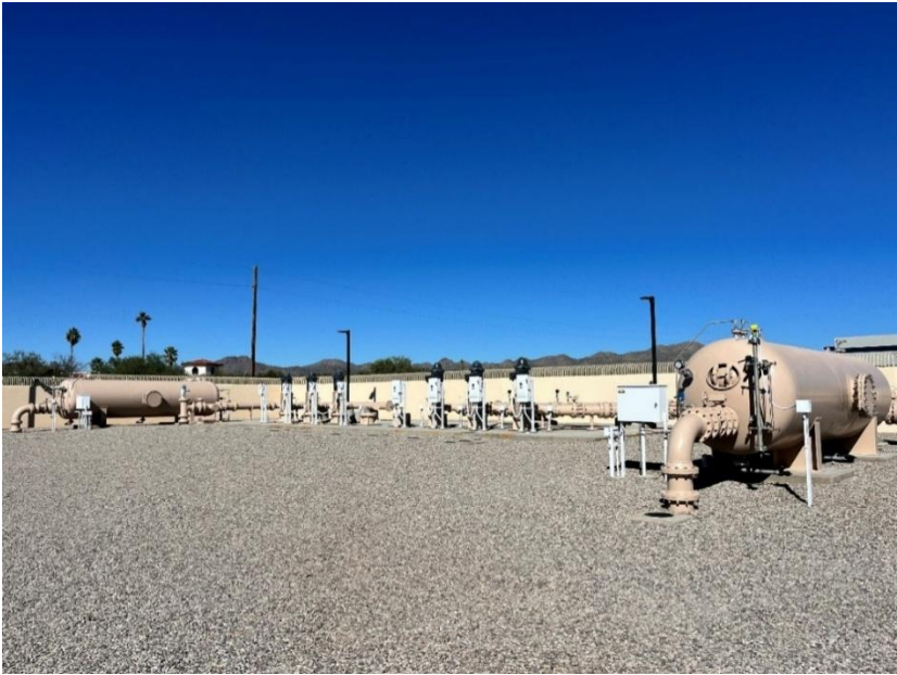
Two Zone Booster Site at La Canada. Left side of photo is “F” Zone and Right side is “G” Zone.
