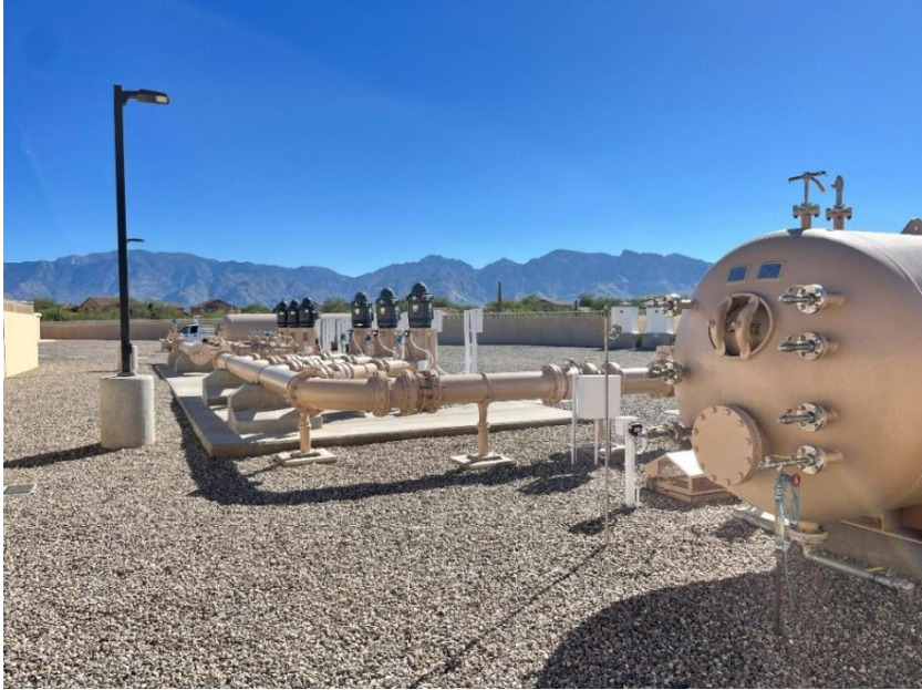
“F” Zone discharge header pipe with meter and 5000 Gallon HP Tank in foreground.
