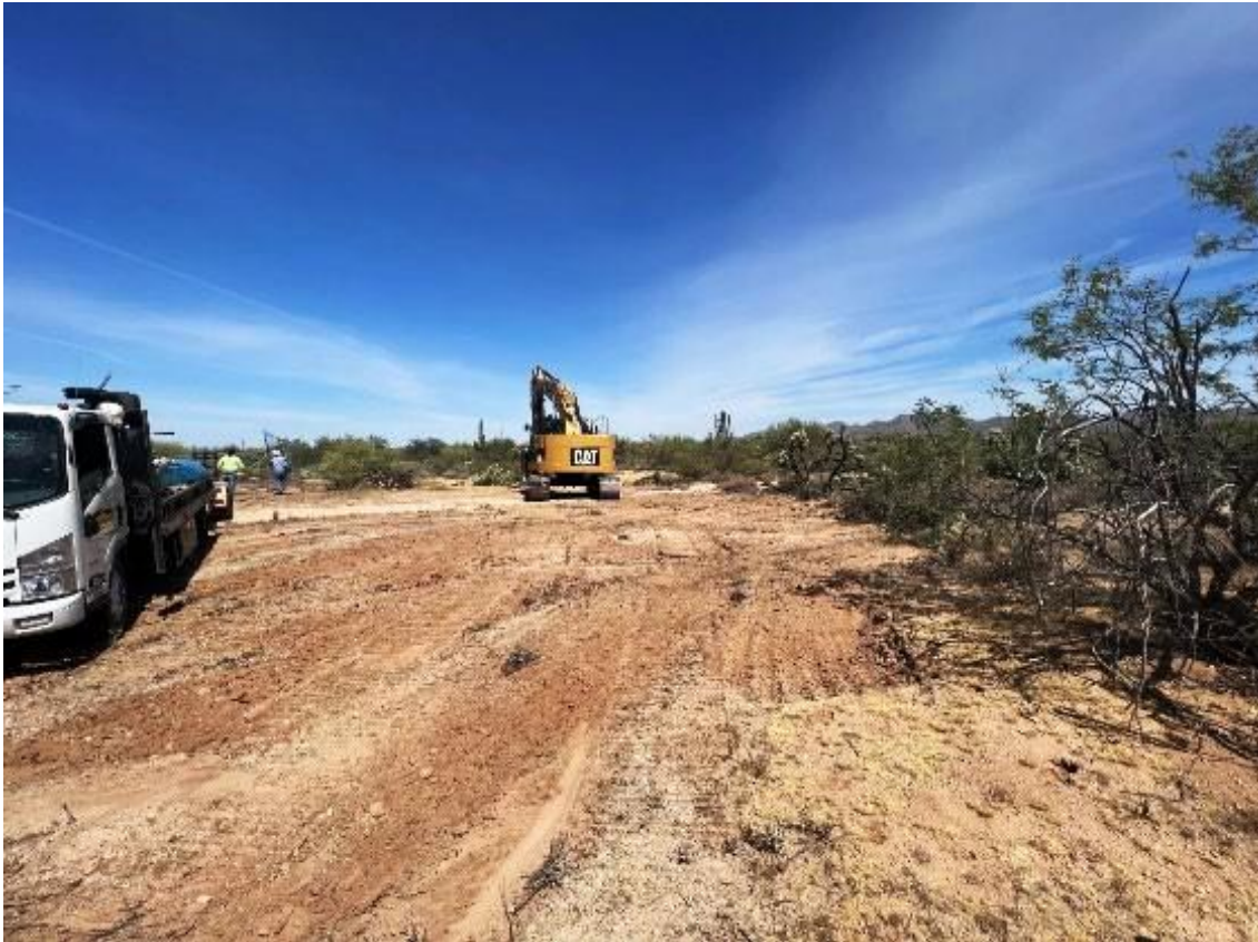
View of the construction of the NWRRDS Independent Shannon Road Booster Station Discharge Main to Tangerine Rd.
