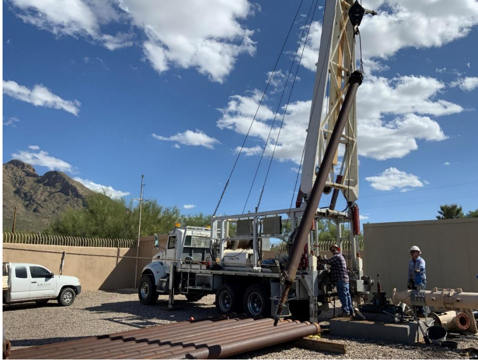
The photo above shows contractor pulling column pipe and pump from Well D-9. Work includes well rehabilitation, vertical turbine pump, and Hi Thrust Motor 200HP
