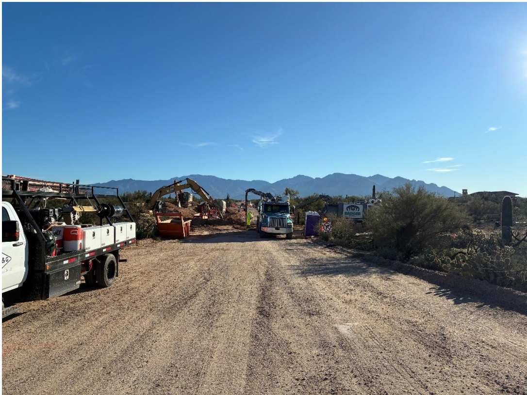
The NWRRDS Independent 20-inch Transmission Main looking east towards the Santa Catalina Mountains at intersection of Camino Del Norte and Oldfather Road
