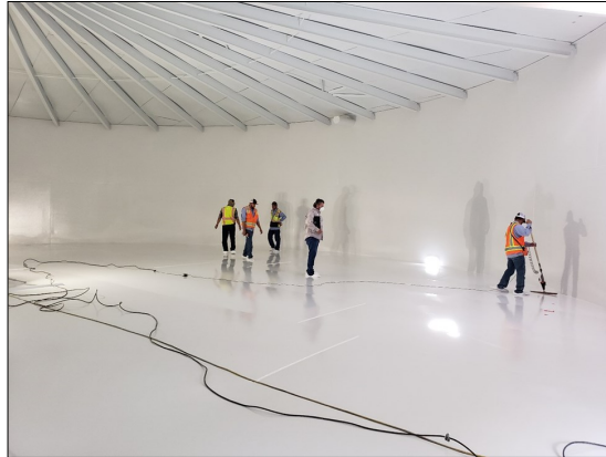
Smyth Industries performs quality control testing on the new lining. The 500,000 gallon reservoir was drained, sandblasted, repaired, cleaned and relined.
