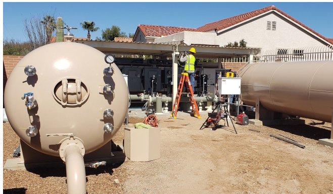
The Rancho Vistoso Booster Station nears completion. The testing and final acceptance of the facility will take place in March. The construction cost will be $417,000. Infrastructure investments like this are necessary to ensure a safe and reliable water system.
