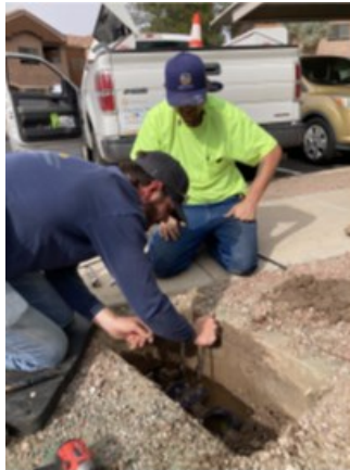
Meter Operations staff are shown replacing a meter at an apartment complex. Staff perform this type of work daily every day of the workweek.
