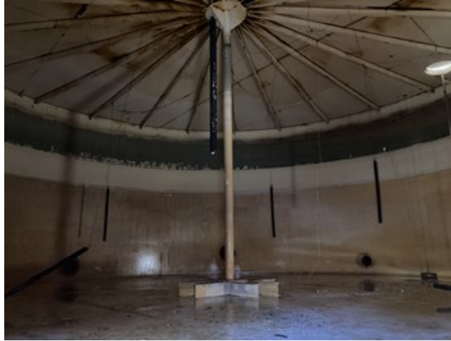
This photograph shows the Big Wash 200,000 gallon reservoir after it was drained prior to sand blasting. The reservoir showed signs that it was past due for rehabilitation work.
