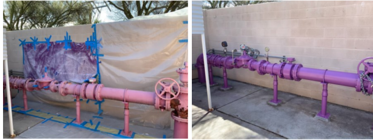
A before and after photo of the kind of work performed by the Utility's ADC workers.
