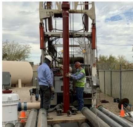
a contractor installs a new pump in one of two wells slated for rehabilitation this fiscal year.
