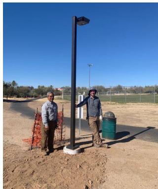
Riverfront Park Solar Lights
