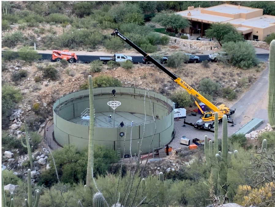
(Above) The construction staff of Smyth Industries completes the installation of the perimeter walls of the new Allied Signal Reservoir. Approximately $750,000 of the Utility's $6 million 2018 bond proceeds are funding this capital investment effort.
