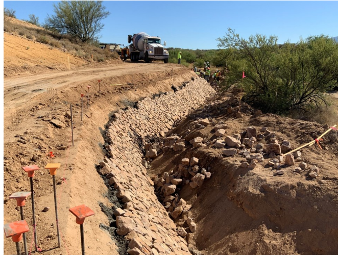
The Water Utility contracted with Borderland Construction Company to construct the slope stabilization elements for the Nakoma Sky well site.
