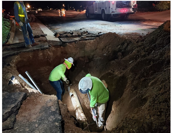
Oro Valley Water Utility Staff expose the 8-inch PVC water main to determine the limits of the damage and to prepare for a section of the existing water mains removal and replacement.
