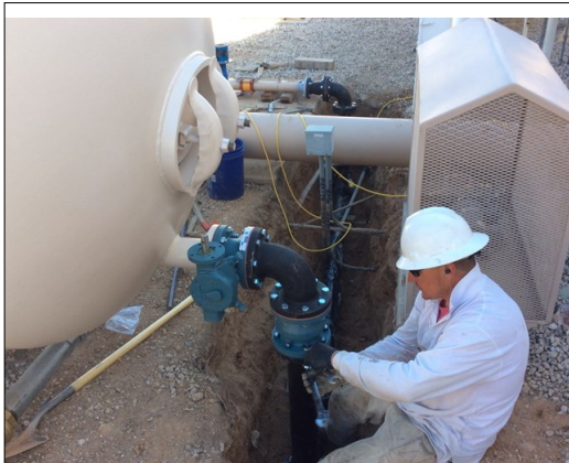
The contractor assembles buried piping as part of the installation of a new ASME certified pressure vessel.
