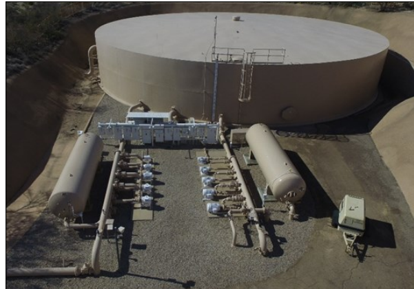
The Water Utility's High Mesa Reservoir and Booster station pictured above. Replacement of a non-ASME certified pressure vessel and booster station modifications were performed as part of the Utility's ongoing Capital program.
