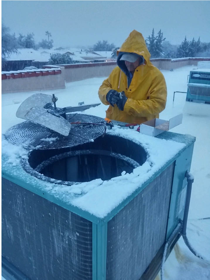
Rain or shine, PW Maintenance ensures the Town Hall Buildings' Air Conditioning is ready for use
